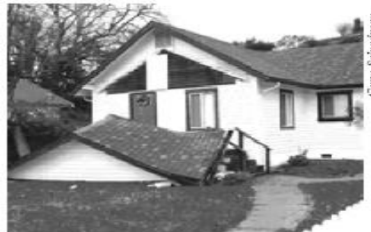
Figure 6 - San Simeon Earthquake, Dec. 22, 2003 The collapsed porch was not adequately attached to this single family residence.
