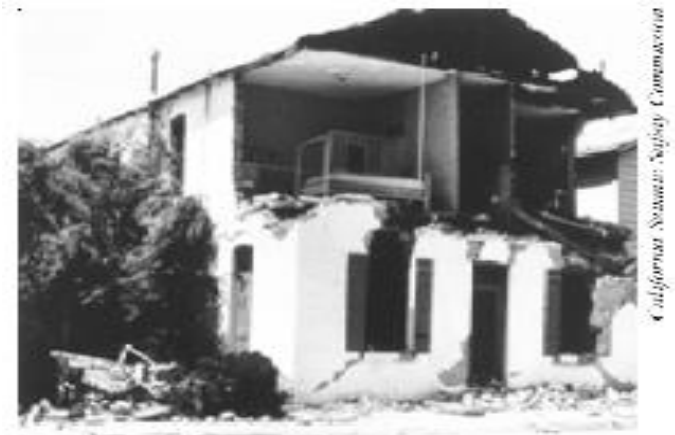
Figure 25 - The plaster-covered brick walls of this building collapsed during a recent earthquake.
