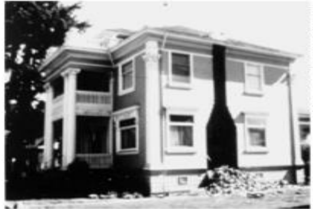
Figure 33 - This unreinforced chimney fell during a recent earthquake.
