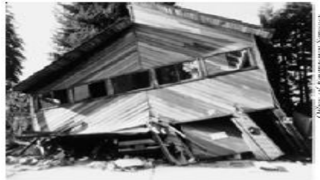
Figure 29 - This mountain home was built over a garage, and its walls were not strong enough to withstand an earthquake.
