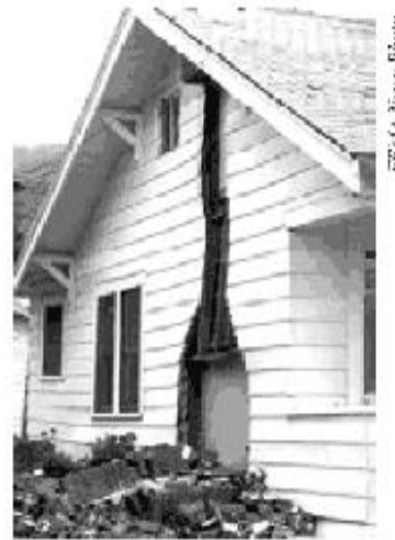
Figure 4 -Northridge Earthquake, Jan. 17, 1994 Chimney Collapse - common type of damage to unreinforced masonry.
