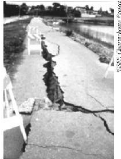
Figure 39 - Lateral Spreading. Loma Prieta Earthquake, October 17, 1989. Lateral spreading damage levee road along the San Lorenzo River.
