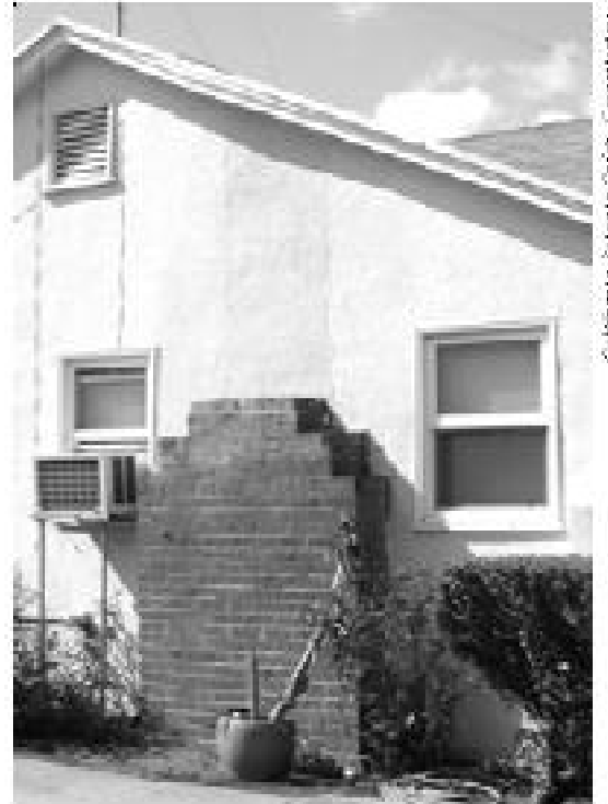
Figure 35 - Photo showing damaged chimney removed. Note that the fireplace is now not functional.
