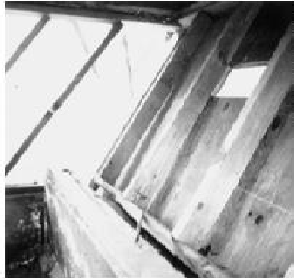
Figure 23 - This photograph shows an interior detail of a home similar to the one above, showing substantial damage to a building with an unbraced tall wall.
