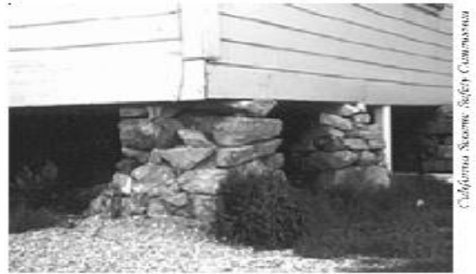
Figure 19 - This is an unreinforced stone foundation. They typically fail during earthquakes.
